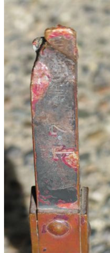
Burnt Lightning Air Terminal 2
